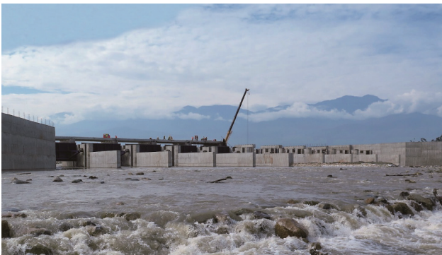
厄瓜多尔可尼尔防洪工程 Canar Flood Control Project, Ecuador –headgates
